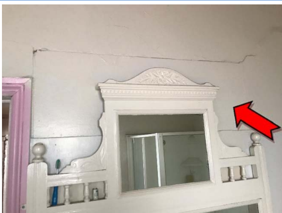
Photo 5. Interior, bathroom, wall panels – asbestos-containing fibre cement sheeting.
