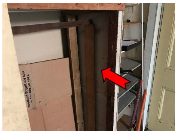
Photo 6. Interior, room 4, wall panels – asbestos-containing fibre cement sheeting.
