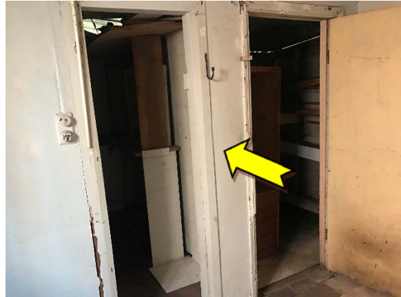
Photo 8. Interior, throughout, wall - suspected lead-containing white upper paint system.
