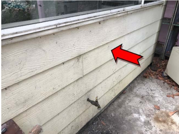
Photo 1. Exterior, northern and eastern elevation, wall cladding – non asbestos-containing fibre cement sheeting.
